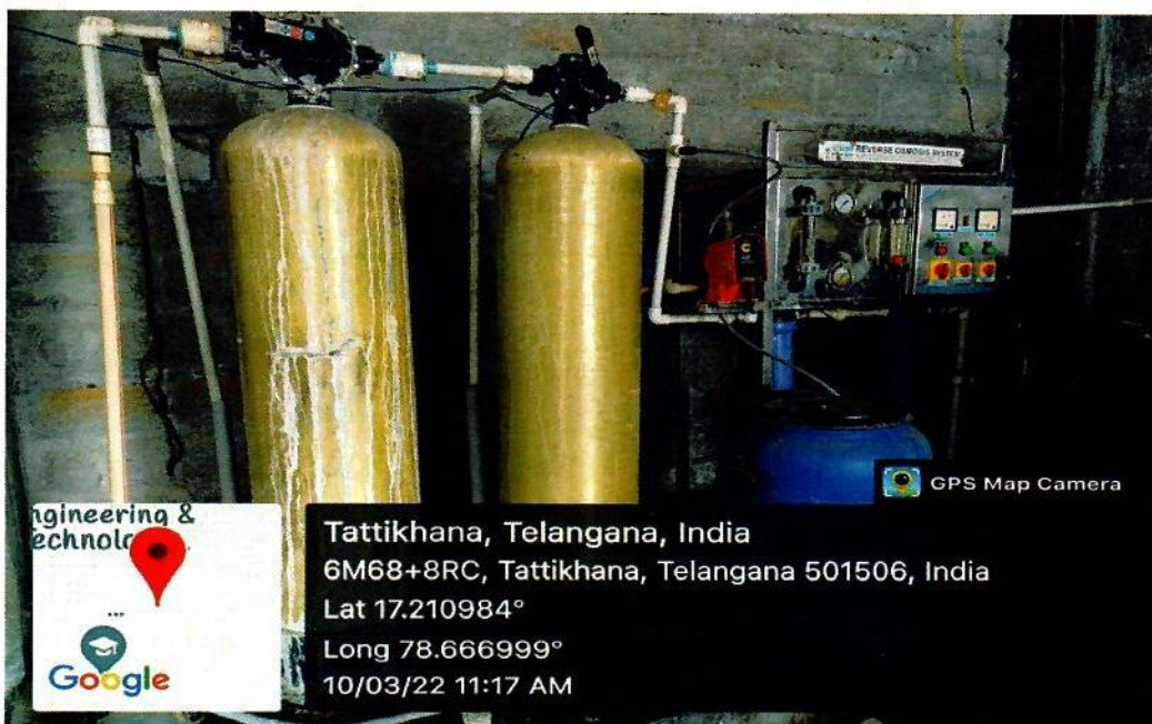
Ro plant in boy's hostel
