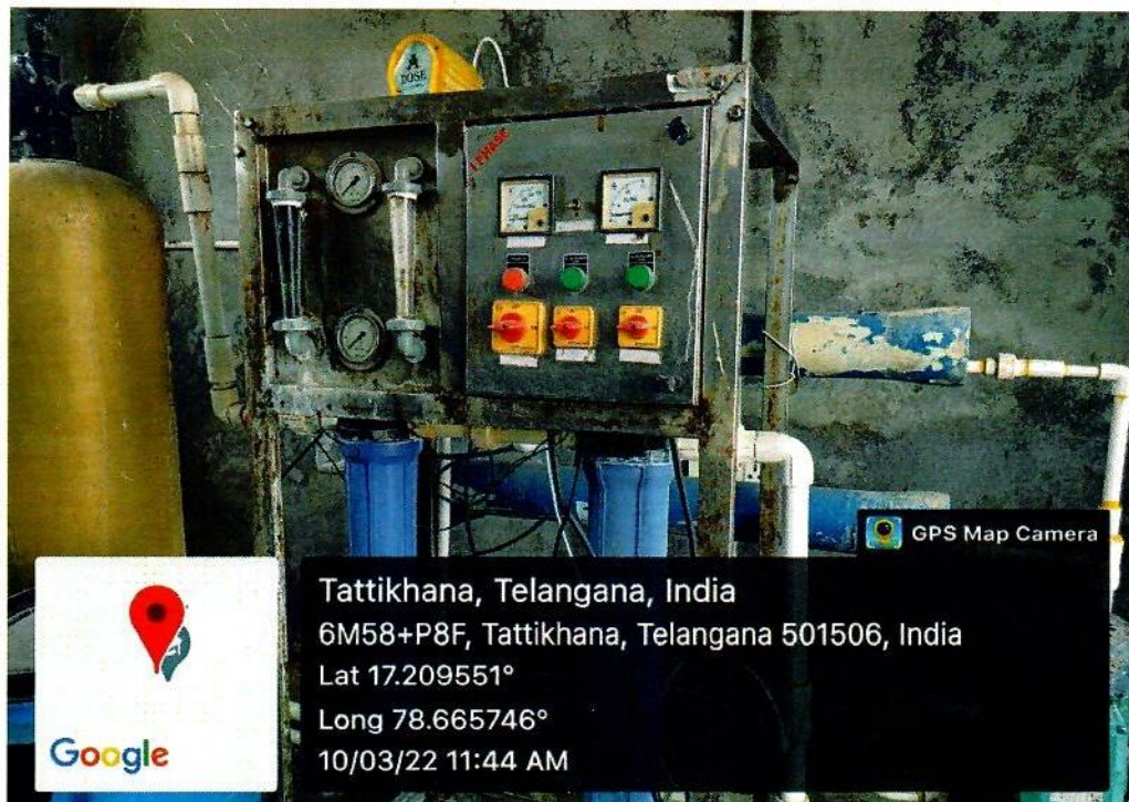
Ro plant in main block
