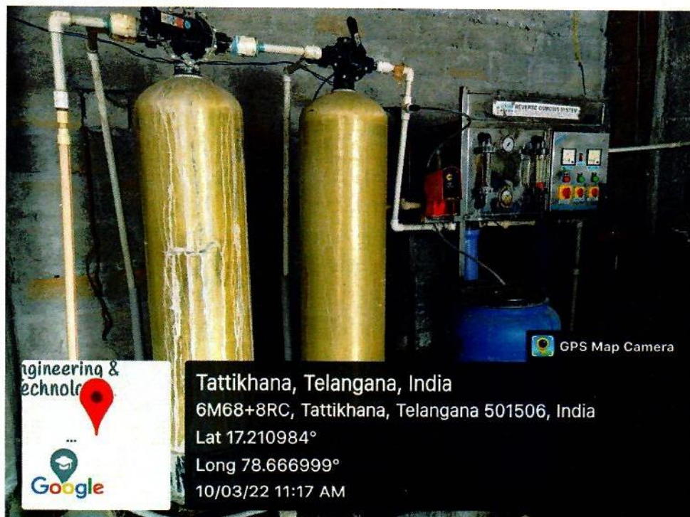
RO Water plant in Boys hostel
