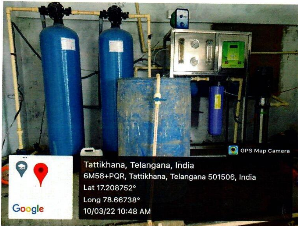
RO Water plant in Girls hostel
