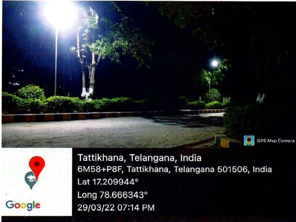
Sensor-based street lights in the campus.
