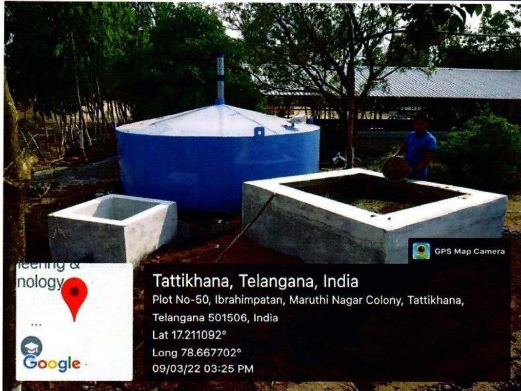
Biogas plant with food waste input.
