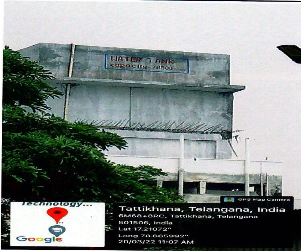
Overhead tank on Boys hostel.
