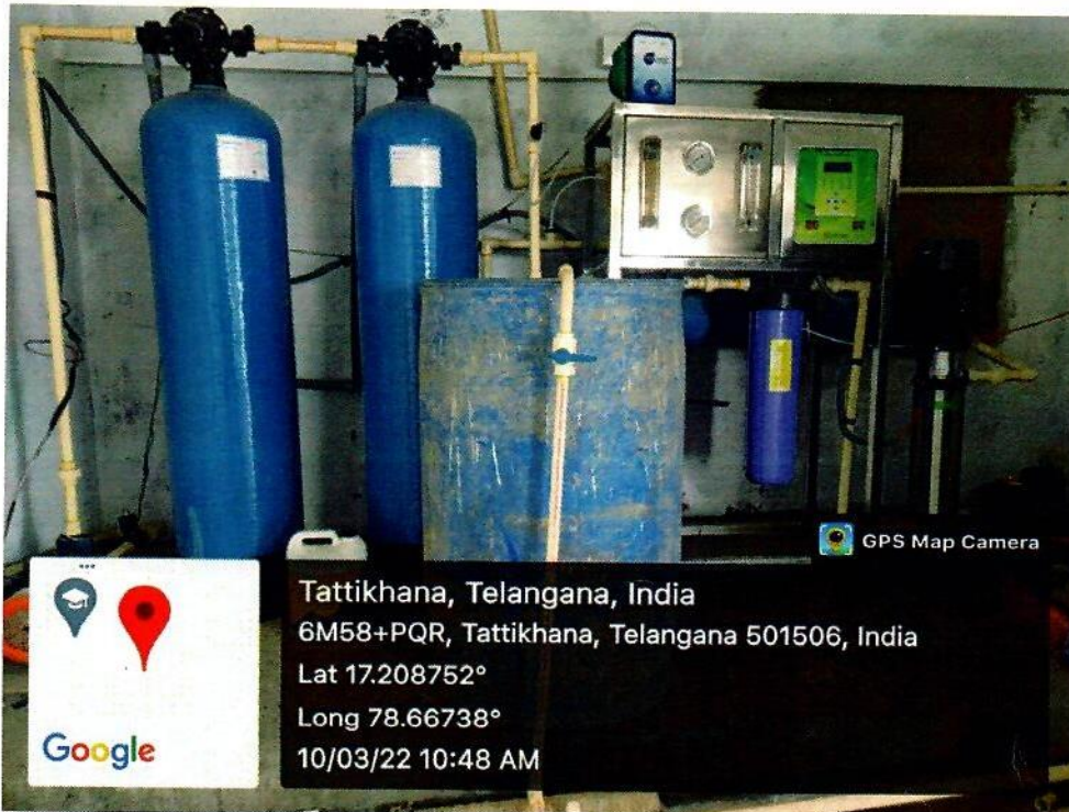
RO Water plant in Girls hostel
